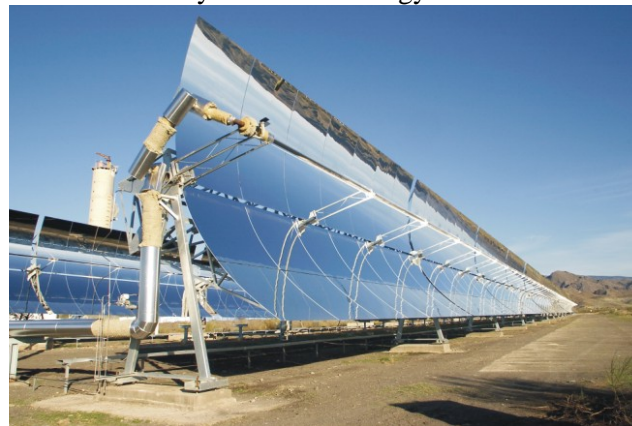
Figure 1: Parabolic trough collectors at solar test center near Almeria, Spain.
